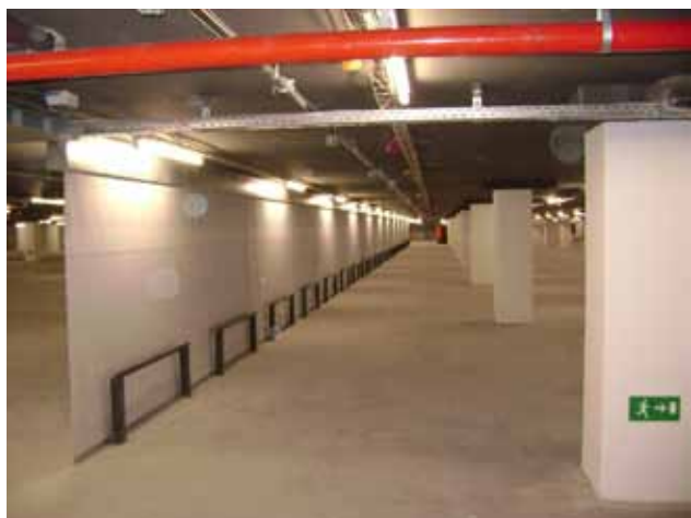
Compartmentering door rookgordijn
